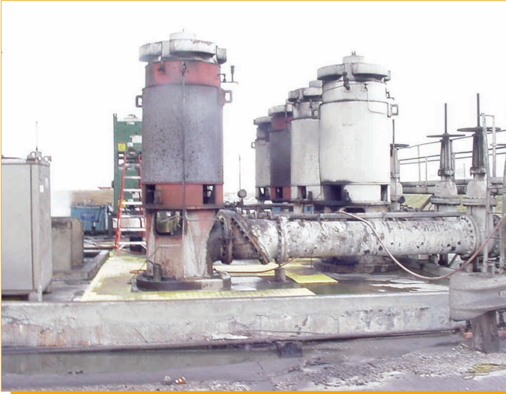
The vertical cooling tower is one of a group that ran bronze bushings and only lasted six months. Composite wear components were installed and several of these have been in service for over three years.
